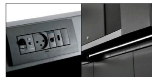
Energy and power supply, LED lighting.
